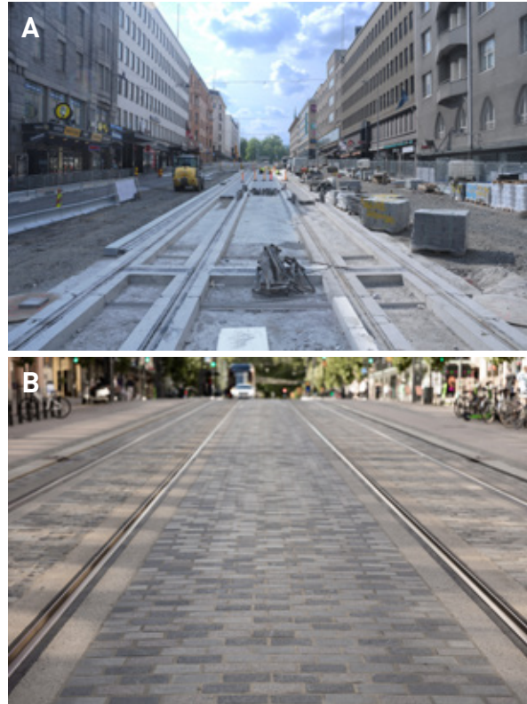
Figure 19. A. Construction of the Tampere tramway at the Hämeenkatu Street in 2018. B. The surface of the superstructure of the tramway is constructed from granites from the Kuru granite quarry district ( Kuru Grey, Kuru Redbrown, Kuru Black ) at the Hämeenkatu Street (2023). See also Cover Photo. Photos: Tampereen Kovakivi Oy.
