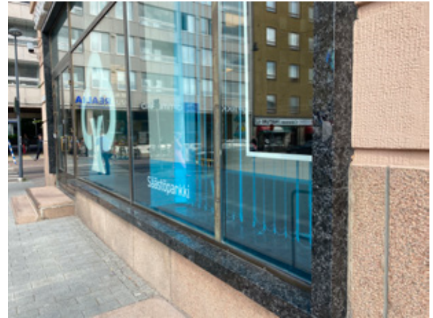
Figure 5. The window frames of the office building Torinkulma. Spectrolite. Photo: Olavi Selonen.
