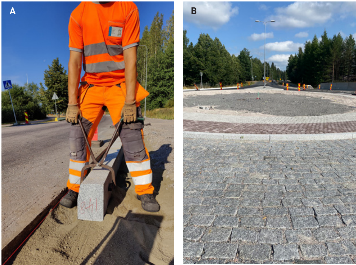
Figure 8. A. Installation of kerbstones along the Helsingintie Street in 2022. B. Roundabout at the Helsingintie Street in 2022. The grey granite from Ristijärvi ( Ristijärvi Grey ) is applied. Photos A: Sini Laine, B: Olavi Selonen.
