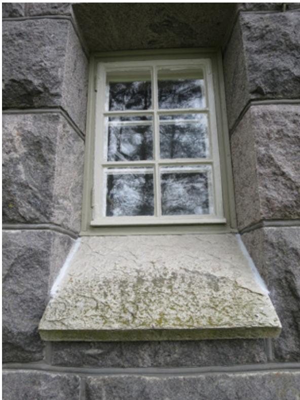
Figure 3. The window sheets in the Varpaisjärvi church are made of Nilsjä quartzite. Photo: Olavi Selonen.
